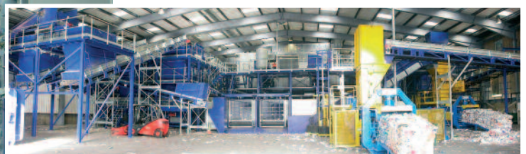
Turn-key solutions maximise recycling rates (Stadler CoMingled Recycling Plant)
